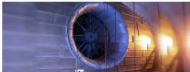
2001: STROMSAS TUNNEL, NORWAY A large axial flow fan of a diameter of 6 meters long was deployed.
