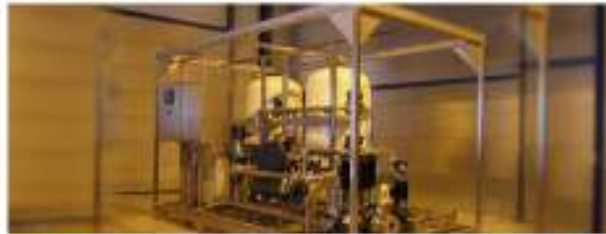
1999: CHINBU TUNNEL, SOUTH KOREA 2 lanes, 2,800 meters long tunnel in Chinbu, South Korea. Installation started in 1998 and finished in 1999. Bypass installation with a total air cleaning volume of 285 m 3 /s.
